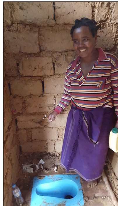
This adaptation of the original SaTo sanitary toilet pan now includes a wider flange. This feature facilitates installations into mud or wood floors, as pictured here in a bathroom in Rwanda.
